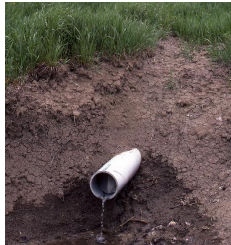
Figure 1: Clean water exiting a modern tile drain.
